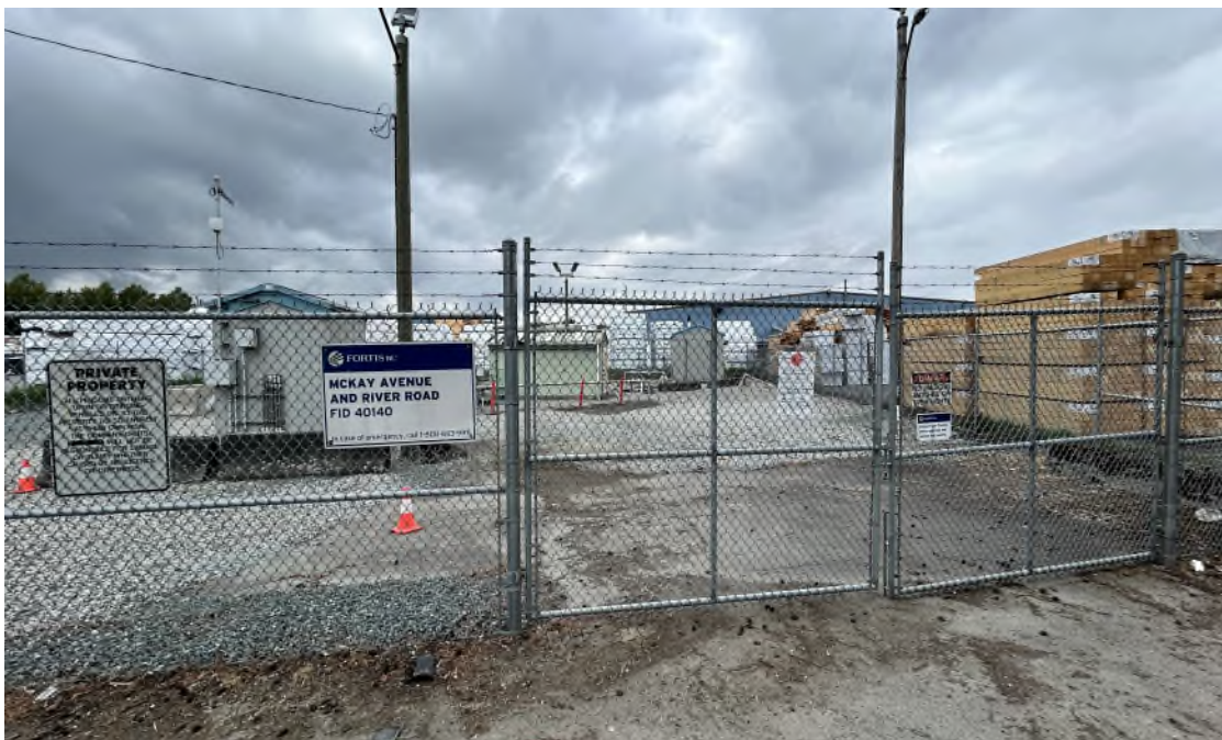
Photo 5 Fortis compression station located on McKay Road, near the intersection with River Road.
