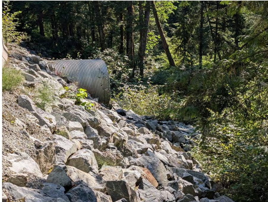
Photo 28: Mapped stream, non-fish passable perched culvert, west of 249 Street.
