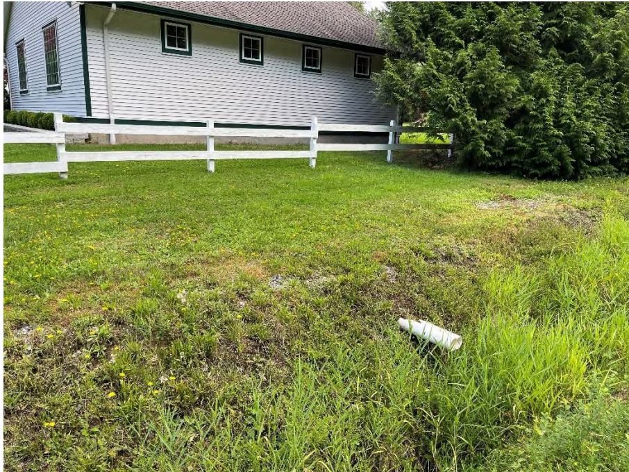
Photo 34: Drain tile outfall into ditch along north side of 130 Ave at 251A Street
