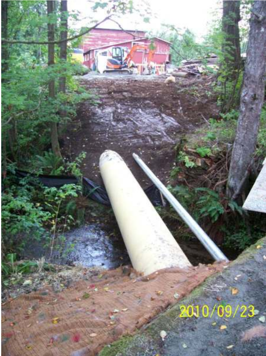
Looking west at Webster Creek aerial crossing showing the casing pipe for the sanitary sewer and galvanized pipe for fibre optic ducts.
