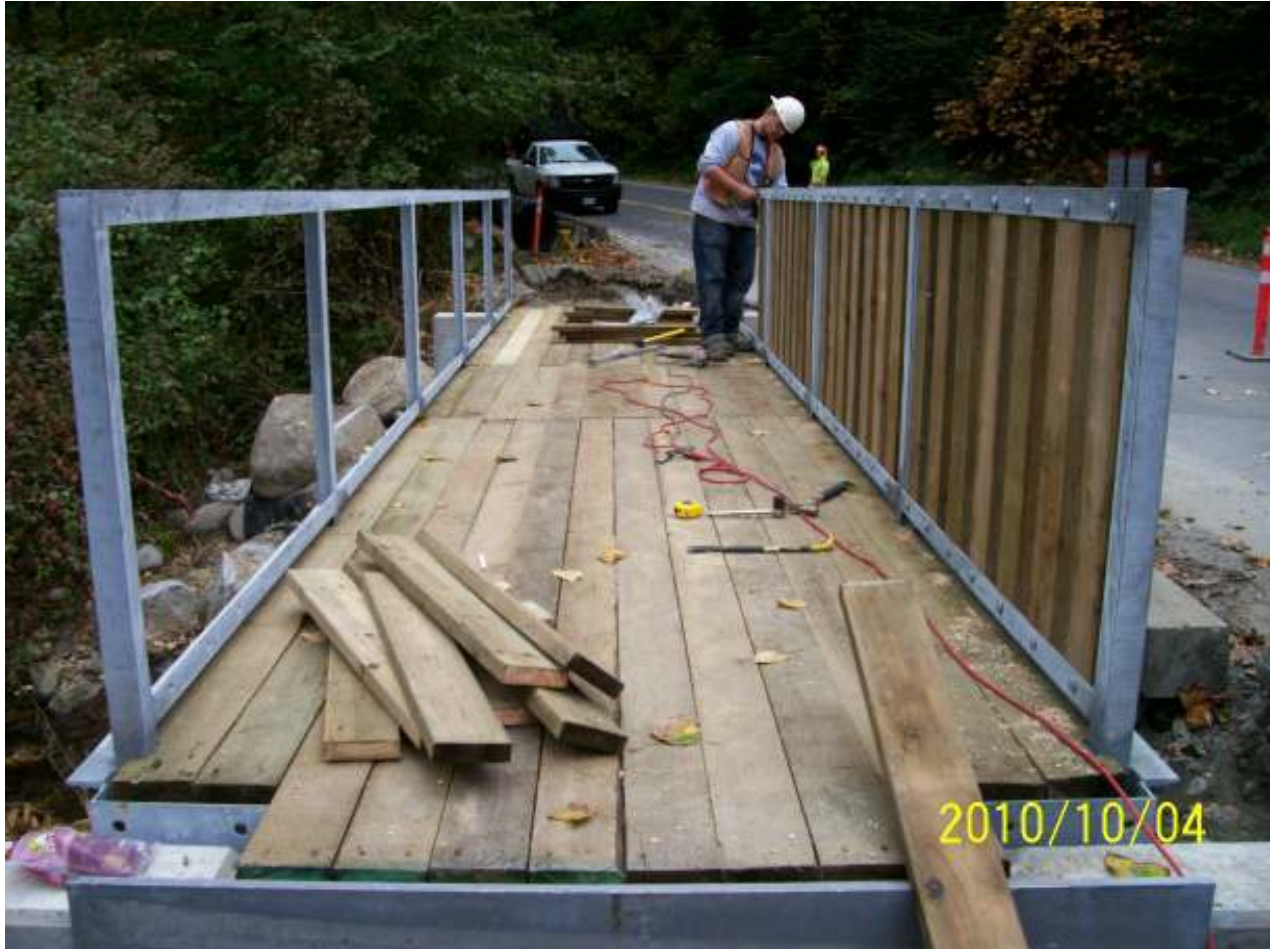
Looking west at Millionaire's Creek crossing. Installing wood planks on the pedestrian bridge above the sanitary sewer aerial crossing.
