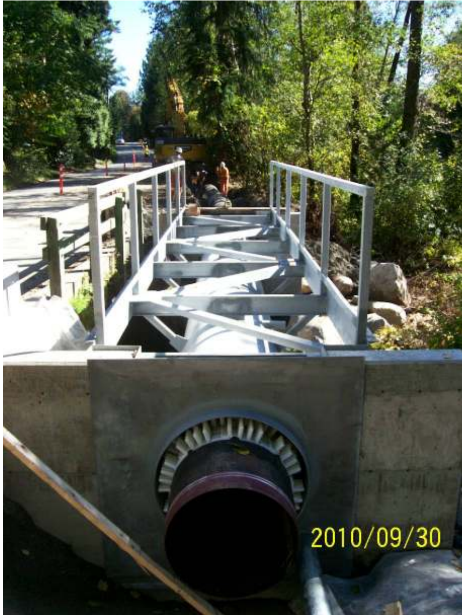
Looking east at Millionaire's Creek crossing showing sanitary sewer pipe inside the casing and under the steel truss pedestrian bridge.
