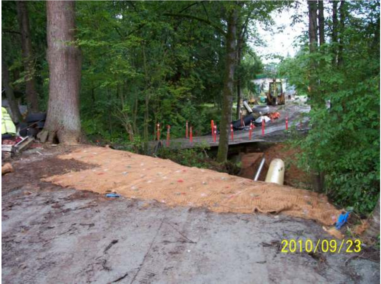
Looking west showing the sanitary sewer route on the 128 Avenue corridor west of 256 Street at Webster Creek crossing.
