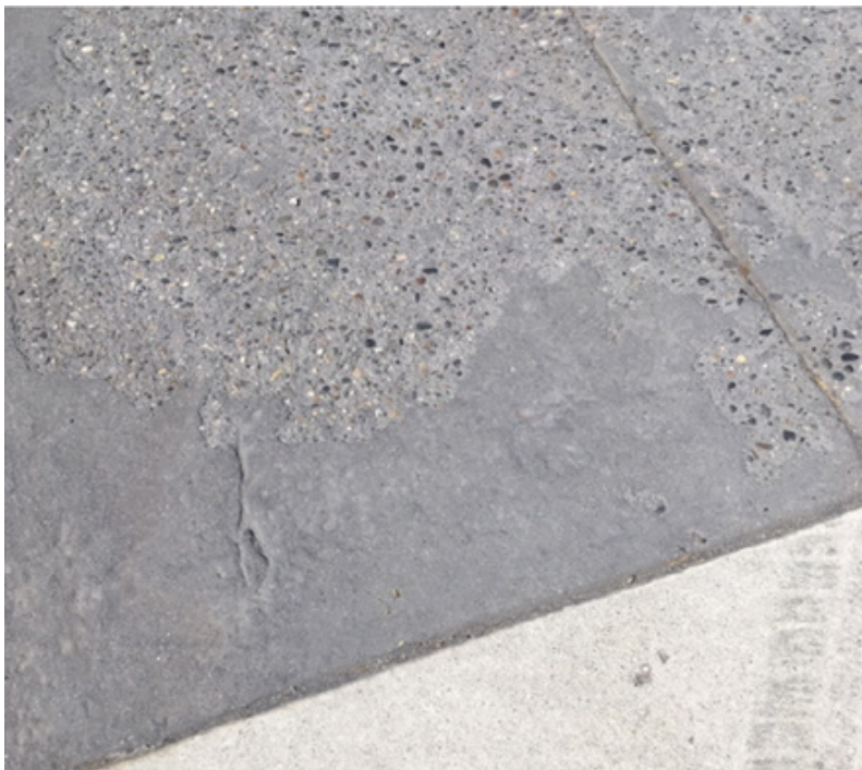
Example of typical salt damage on the concrete sidewalk.
